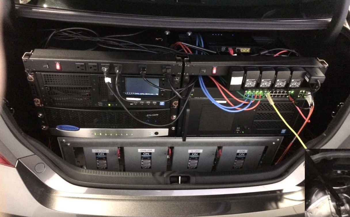
Rear Equipment Bay
